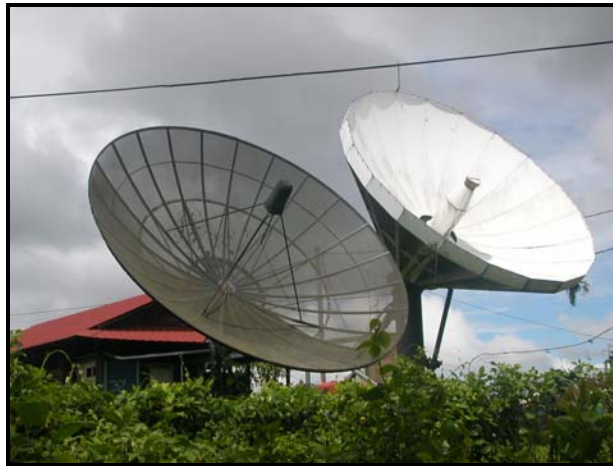
Picture I. Satellite installations at Grand Santi
